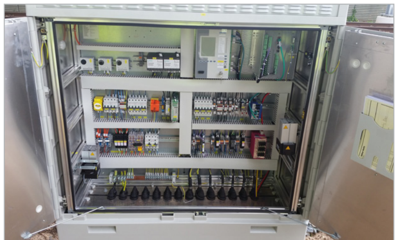
Figure 4: Track-side detection cabinet.
