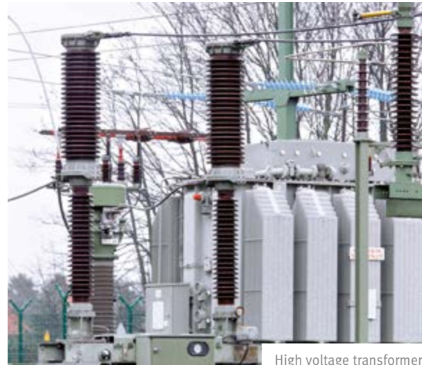
High voltage transformer
