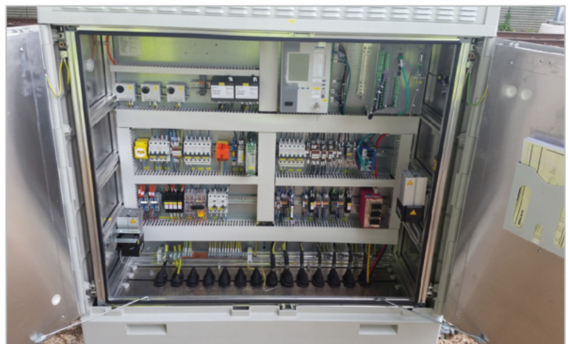
Figure 4: Track-side detection cabinet.
