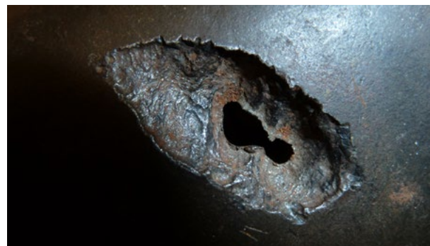
Corrosion damage due to stray currents at a pipework © Ulrich Bette, Institut für Beeinflussungsfragen Wuppertal
