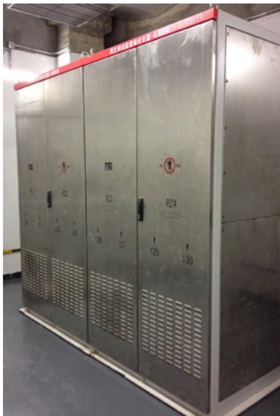
Figure 3: Brake resistor in a substation
