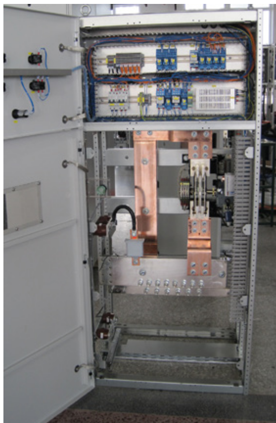
Figure 11: Disconnecter switch panel.
