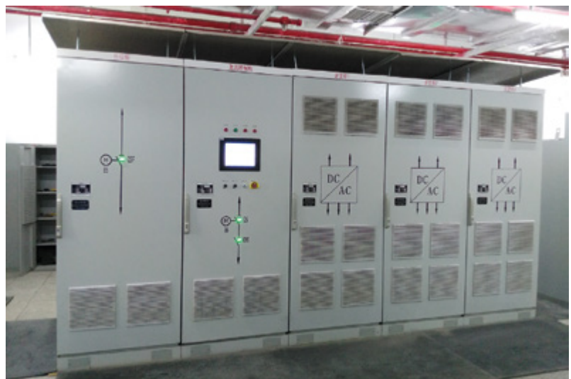
Figure 10: Inverter for recovering braking energy and feeding it back into the medium-voltage system
