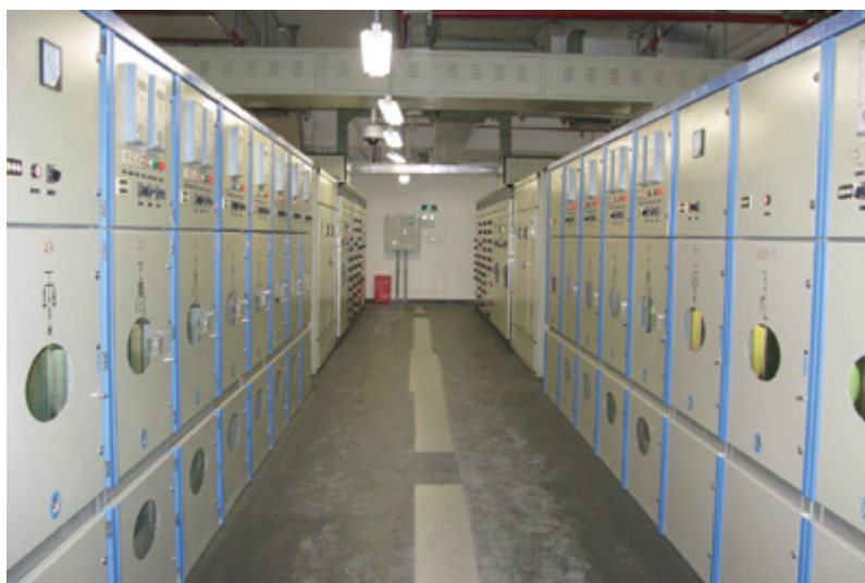
Figure 7: Medium-voltage switchboard 3AC 10 kV 50 Hz in a substation
